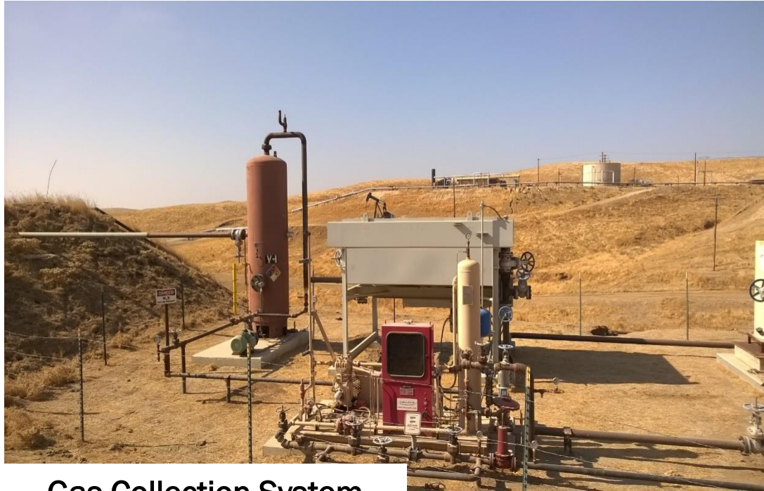
Gas Collection System
