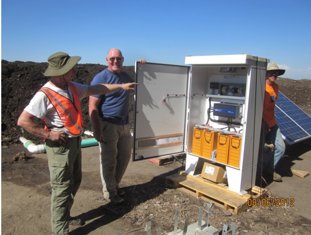
Photo 8: Interior of the power array box. From bottom to top: batteries, inverter, timer and switches, and exhaust fan at very top. From left to right: Harold Ruppert and Peter Moon of 02 Compost, and Kevin Barnes, City of Bakersfield.
