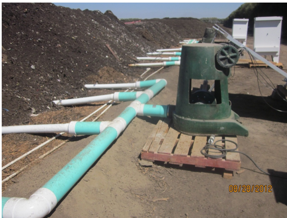
Photo 5: Completed aeration manifold showing 6" pipes, connectors and step down to 4" pipes. The blower is protected inside the modified trash container.
