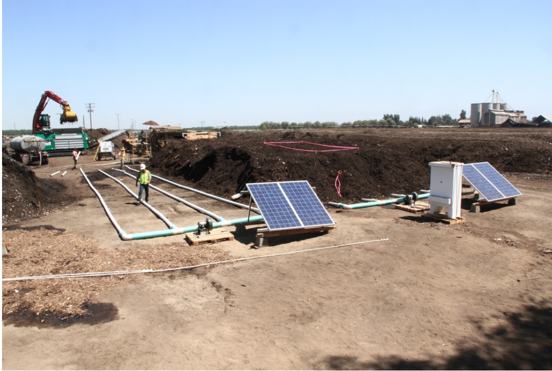
Photo 6: View of project with completed eASP zone 1 on right, and aeration pipes in place for Zone 2. Zone 1 photovoltaic system is complete; panels are in place for Zone 2.
