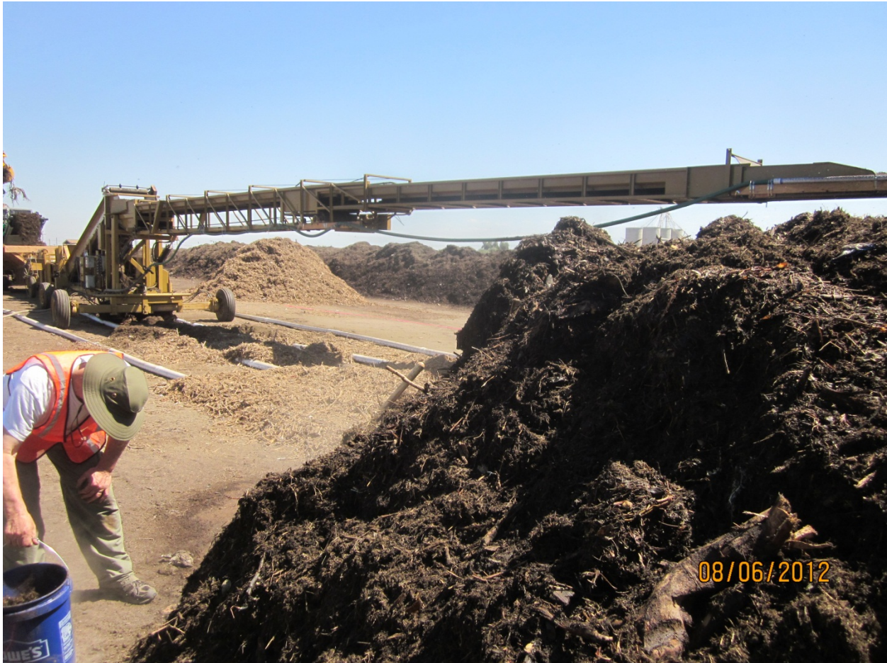
Photo 1: Potato piler at or near full extension. Pile under construction in foreground. Plenum material and aeration pipes are partially visible.
